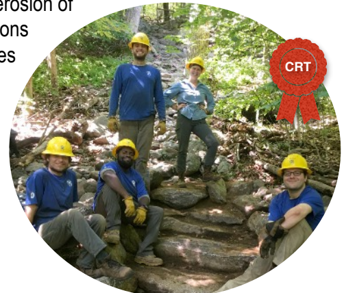
White Dot Trail staircase and crew, NH Photo Credit: Zach Colatch, SCA
