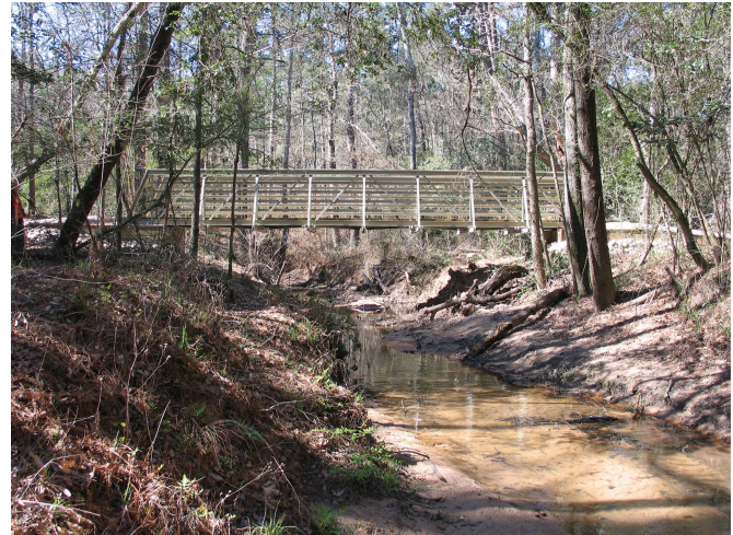
Figure 5—A fiber-reinforced polymer bridge where the truss is also part of the handrail system.
