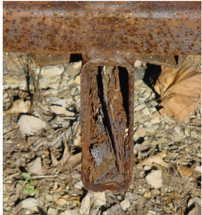
Figure 16—A weathering steel floor beam with corrosion issues in a humid climate.
