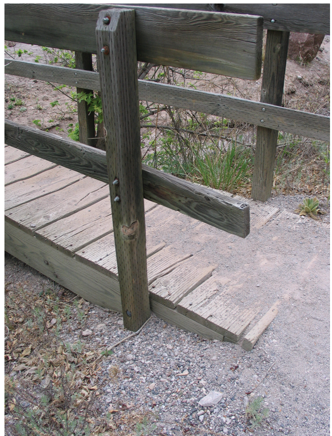
Figure 15—Backwalls should be extended to prevent the soil from contacting the beams.
