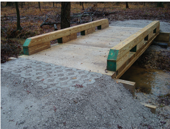
Figure 1—A 15-foot span timber bridge classified as a minor trail bridge, which was constructed using Forest Service standard trail bridge plans.
