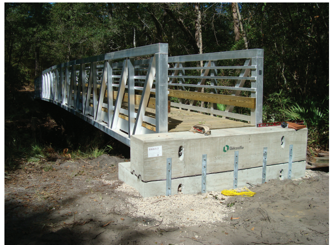
Figure 17—Rub rails installed on an aluminum side truss bridge to protect the railing system.
