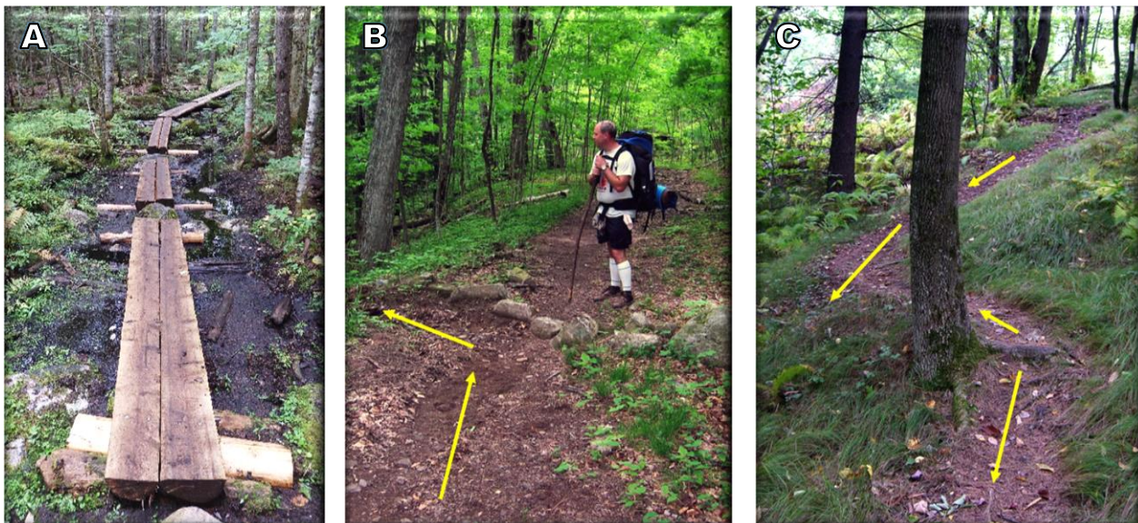
Figure 31. Bog-bridging (A) is an effective practice for raising the tread above wet soils. Rock or wood water bars (knicks) (B) remove water from treads but must be maintained annually to remain effective. Grade reversals of the entire tread (C) will always remove all water and require little to no maintenance.
