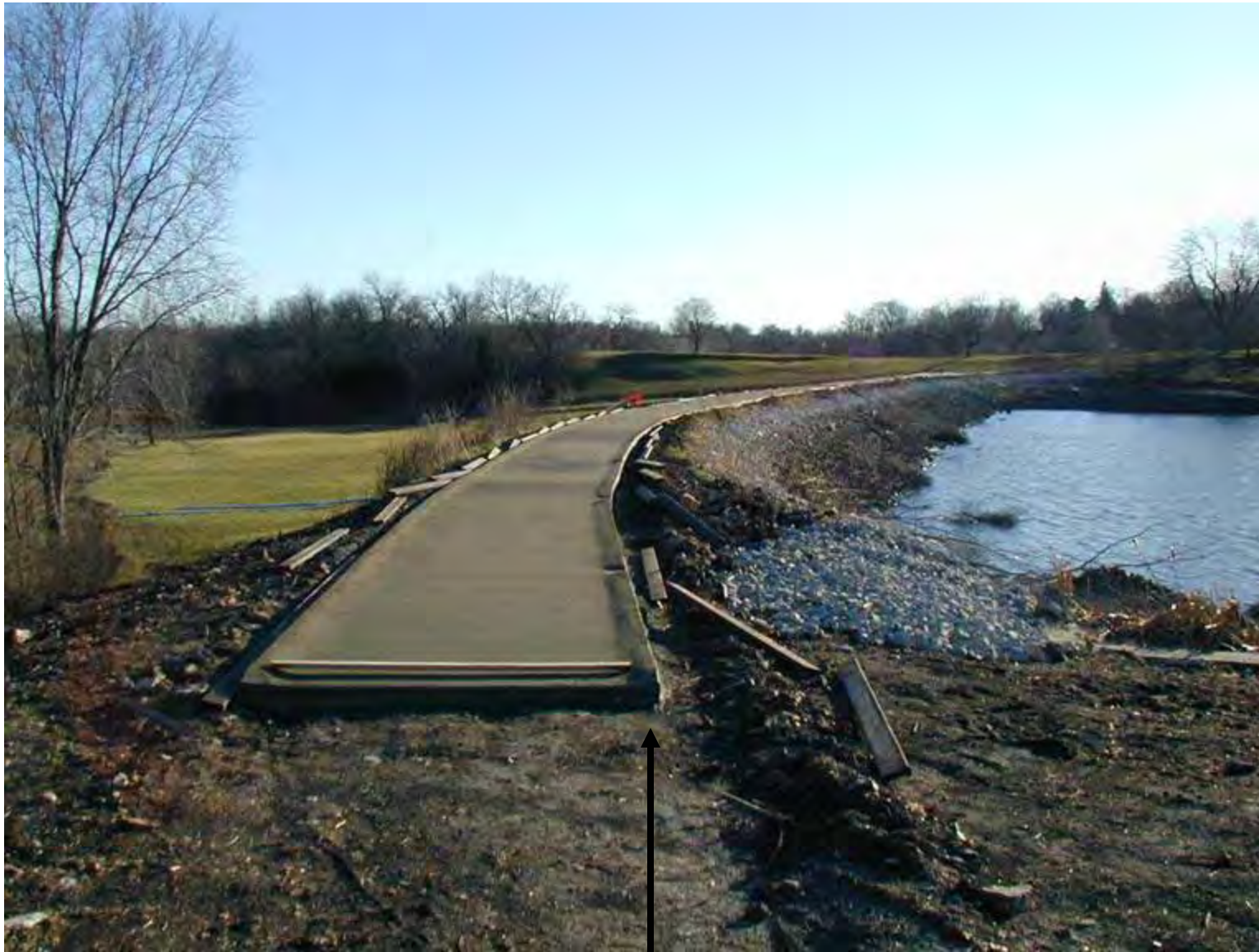
Concrete allows for rolled curb to prevent a wheel chair from rolling down steep slopes.
