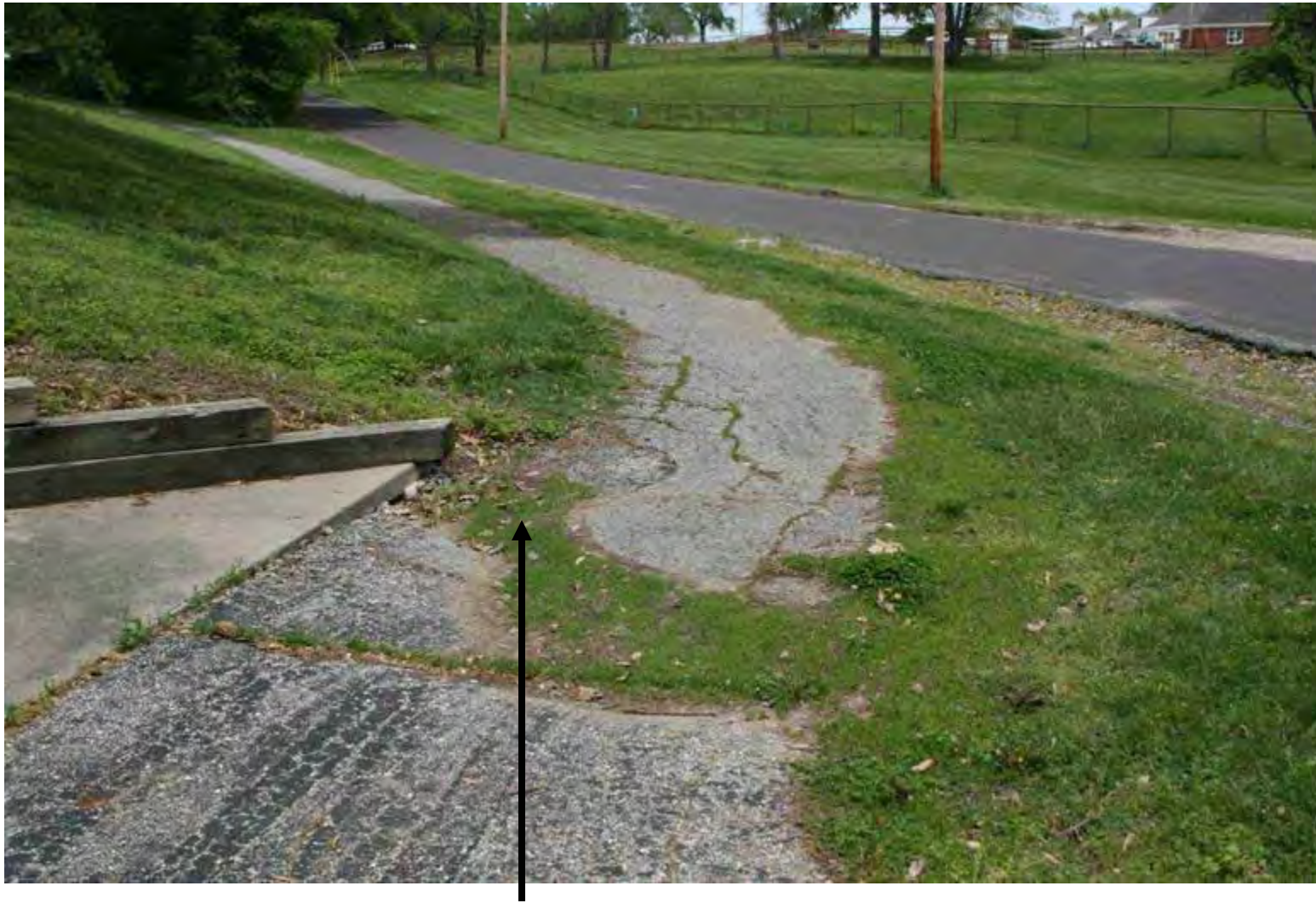
Asphalt settling where base failed on Lions-Stephens Trail.
