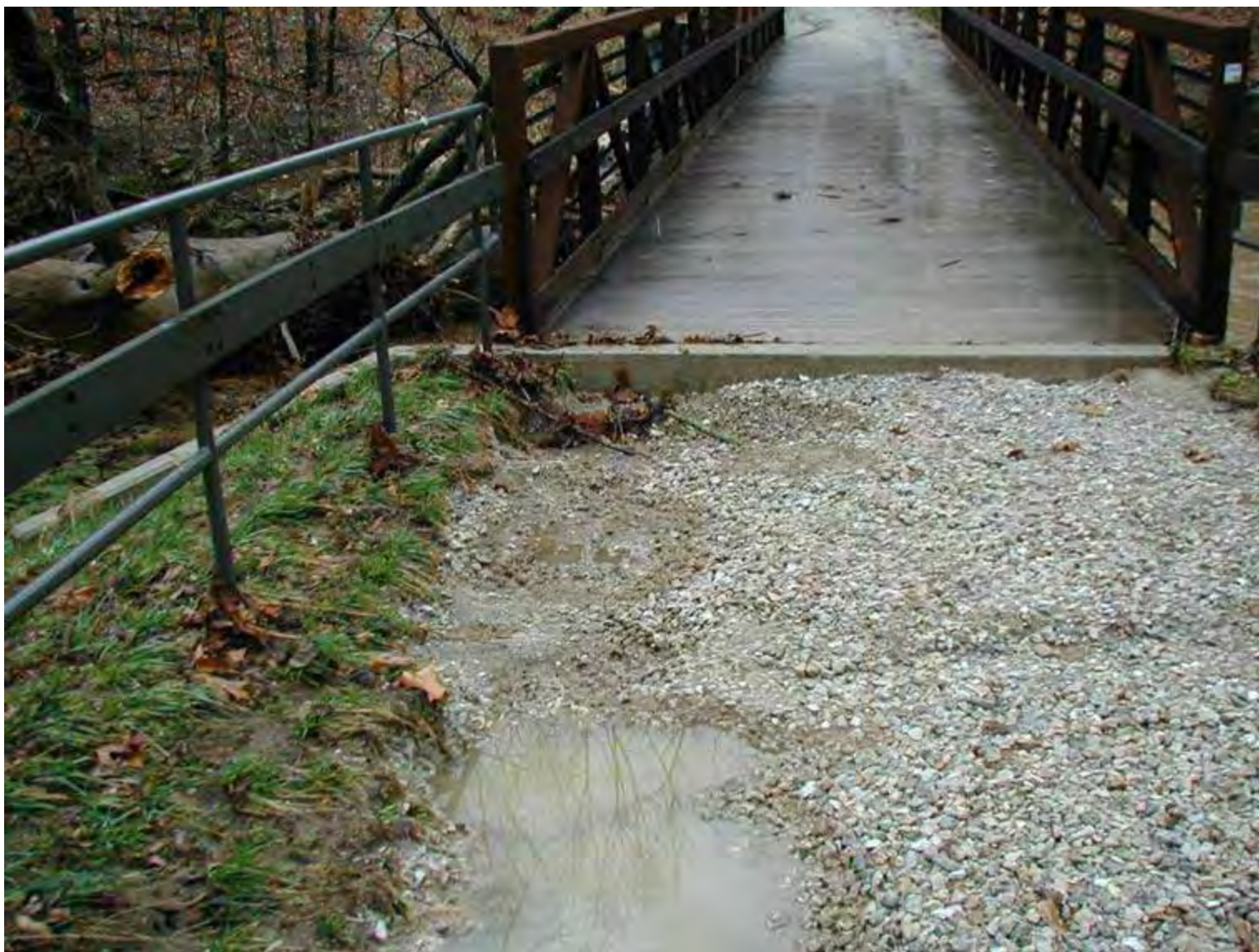
Gravel wash out at Bear Creek Trail bridge.
