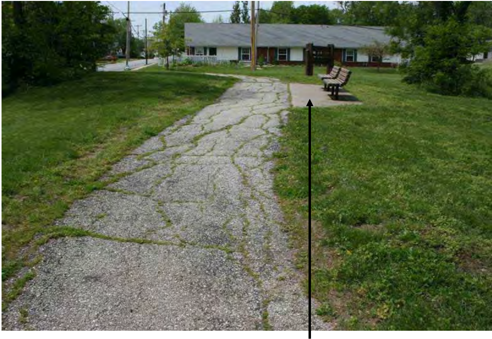
Concrete work done at the same time as asphalt. Lions-Stephens Park 6' wide asphalt trail.
