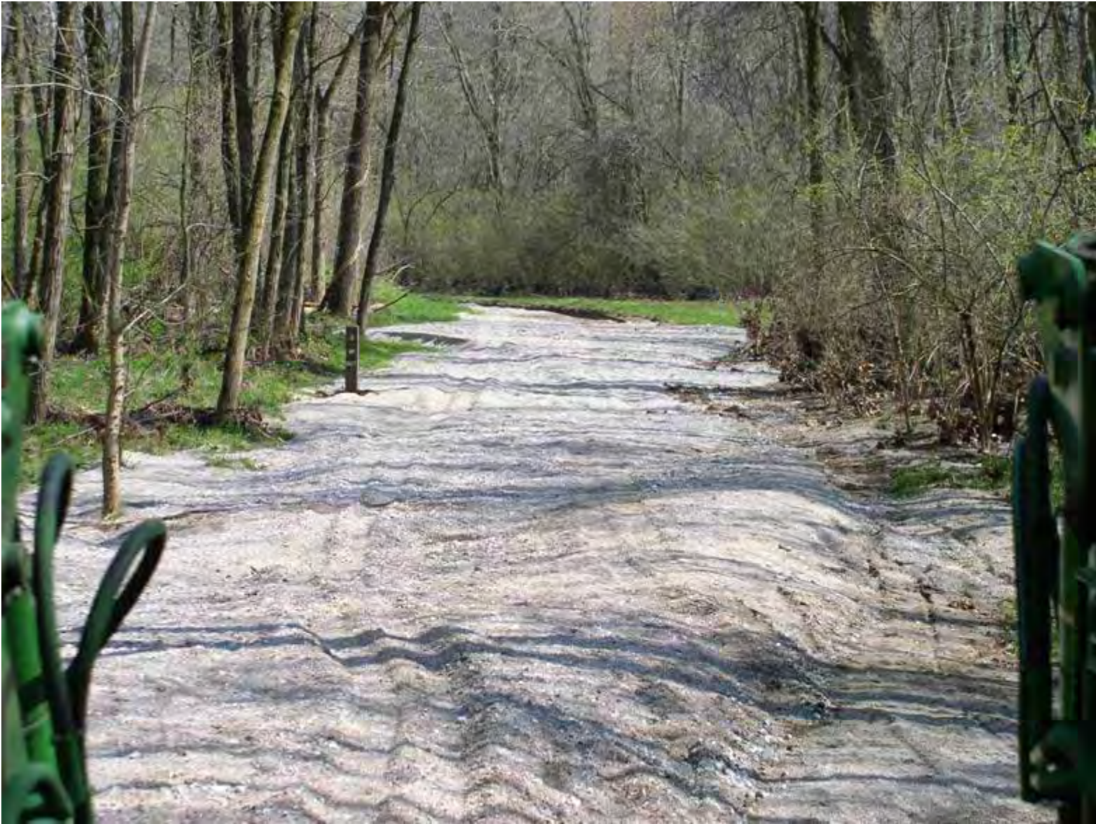
Trail damage after flooding.
