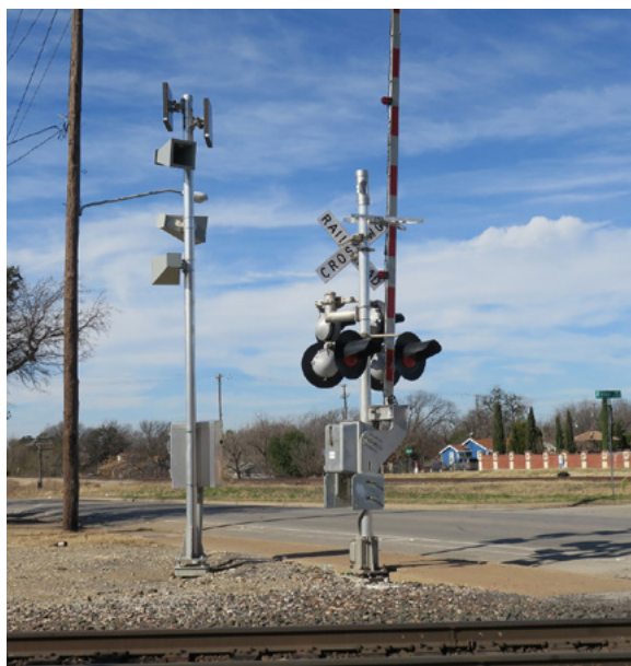
Figure 26. Automated Wayside Horn
