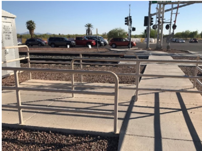
Figure 52. Illustrative Example of a Pedestrian Barrier Application (BNSF Cotton Crossing. Peoria, AZ USDOT 025405Y)
