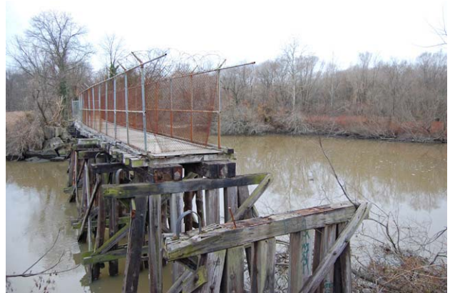
Trail users may use Washington Street bridge rather than restoring this dismantled bridge in Bridgeton
