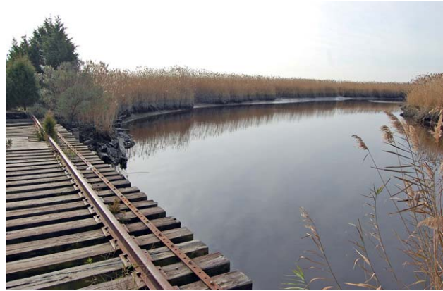
Pennsylvania – Reading Seashore Lines bridge over Muskee Creek in Maurice River Township
