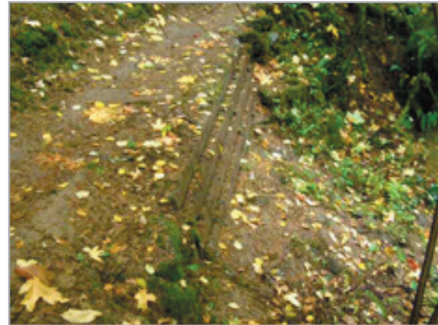
Woods Memorial Natural Area - this cribbed retaining wall helped relocate trail away from edge of creek
