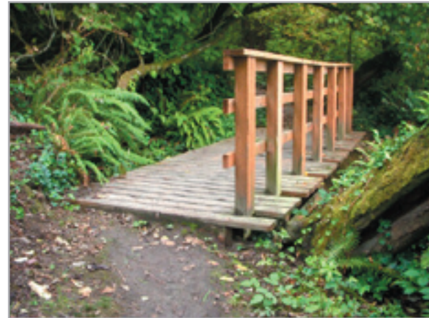
Horizontal railing on side of bridge with minimal fall hazard - Ridge Trail in Forest Park
