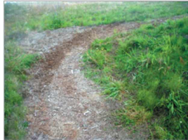
Columbia Slough Trail switchback on west side of cross-levee - grass has grown so vigorously that grasspave material and swale are no longer visible
