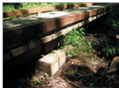
Raz-Baack crossing at Stephens Creek Nature Park - bridge pier block and beam
