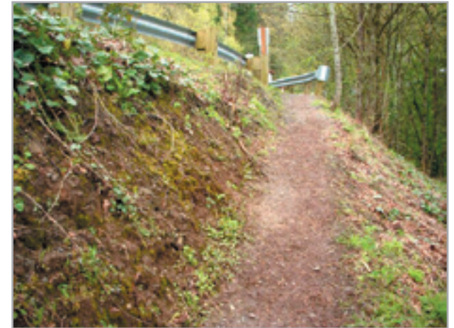
SW Trail #5 at Dickinson Park - steep segment on fill slope of SW 55th Avenue
