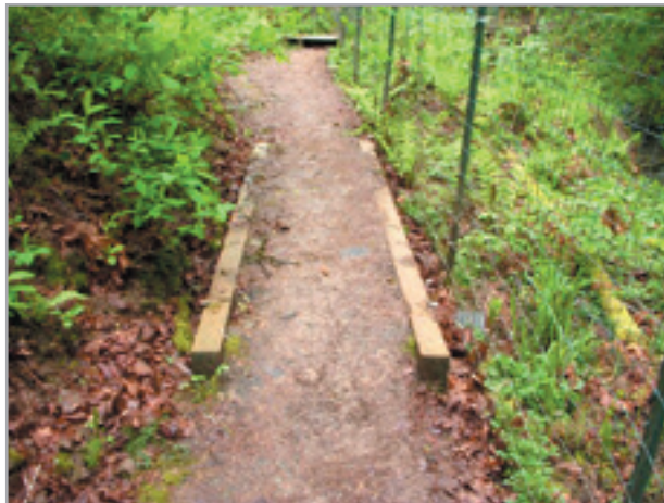
Woods Memorial Park - causeway using 4" x 6" timbers (under construction with temporary metal fence to protect new plantings and prevent trampling of bank of Woods Creek)
