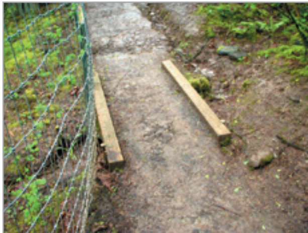
Woods Memorial Park - hiking path (under construction), intercepting runoff in swale and piping under segment of causeway in poorly drained area near Woods Creek
