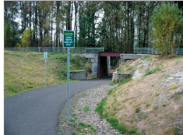
Oaks Bottom Connector at undercrossing to Springwater on the Willamette - infiltration trench on right side
