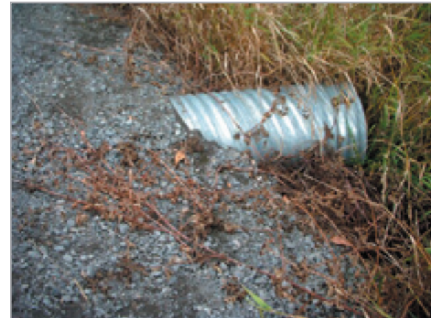
SE 146 Ave connector path to Springwater Corridor (southwest of Powell Butte) right after installation - water in swale next to rail berm and trail flows through corrugated metal pipe, vegetation will grow and obscure pipe
