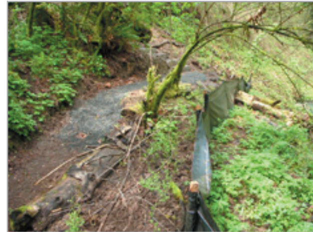
Woods Memorial Natural Area - silt fence between Woods Creek and trail relocation farther from waterway
