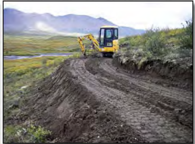
A miniexcavator was used to compact fill slopes, shape backslopes, reduce root wads and place mats of stripped vegetation on exposed soil.
