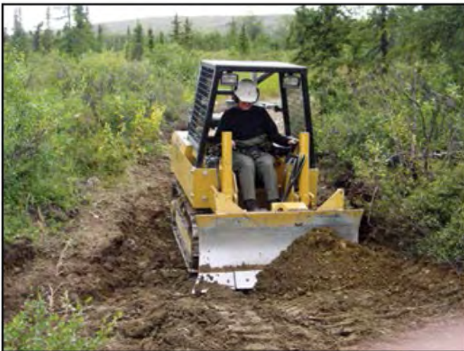
Figure 14–1—A trail dozer is an efficient piece of earth-moving equipment for trail construction and maintenance.
