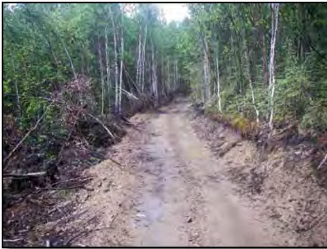
One of the areas where the Sweco 480 was used to directly clear timber from the alignment. Note the trees pushed into the forest.
