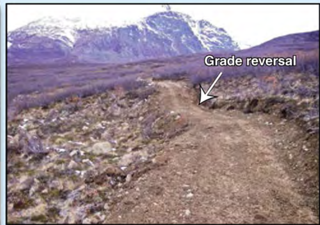
Figure 2–7—Grade reversals are much more effective than waterbars and require less maintenance.
