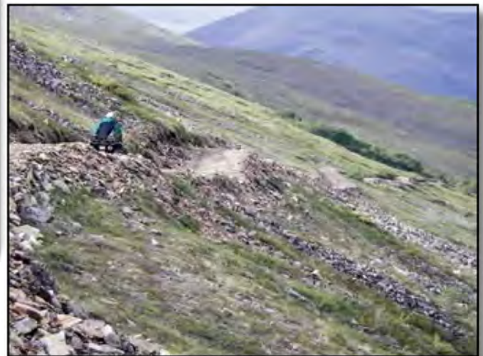
Figure 12-10—This trail displays the stair-step alignment that is characteristic of integrating grade reversals when ascending or descending a sideslope.
