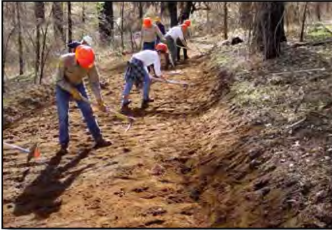
Figure 12-1—A trail crew uses handtools to shape the final tread surface to meet the design specifications.
