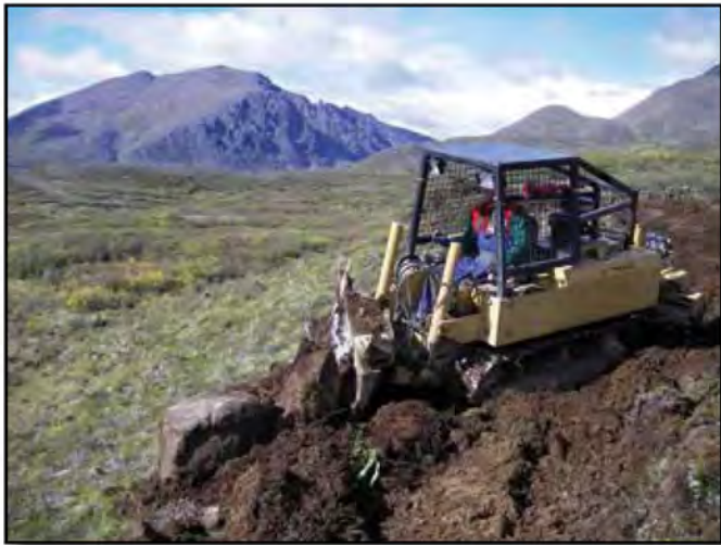
Weighing nearly 10,000 pounds with 83 horsepower, the Sweco 480 (now known as the Sutter 480) is well equipped to handle the many large rocks encountered along the alignment.
