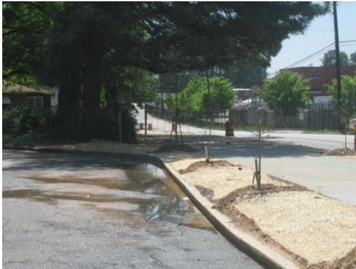
Possible Drainage Issues Associated with Trail Construction.
