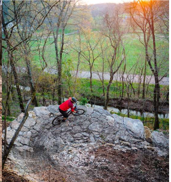
Completed rock berm on Rock Solid at Coler Bike Preserve in Bentonville, Arkansas. Photo by Hansi Johnson
