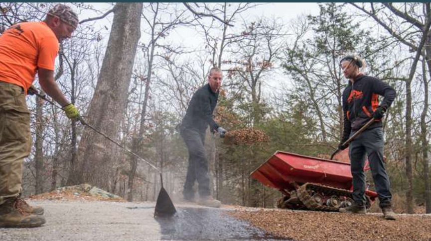
Liquid asphalt and final aggregate coat being applied at Centennial Park in Fayetteville, Arkansas Photo by Eli Glesmann/Rock Solid
