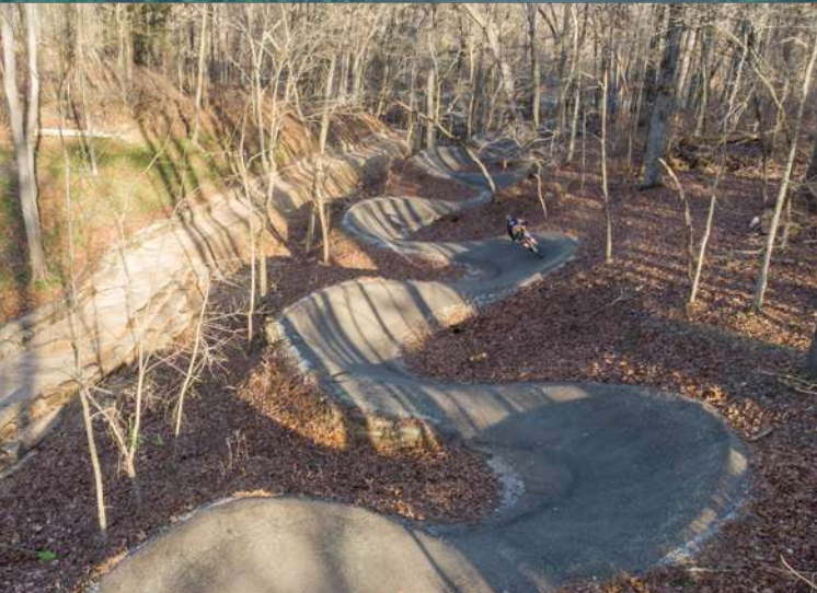
Chip-seal surfaced flowy berm trail at Slaughter Pen in Bentonville, Arkansas. Photo by Eli Glesmann/Rock Solid
