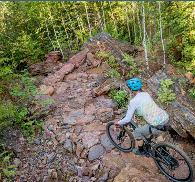
Constructed technical rock tread at Tioga Recreation Area in Cohasset, Minnesota Photo by Chris Guibert/Rock Solid
