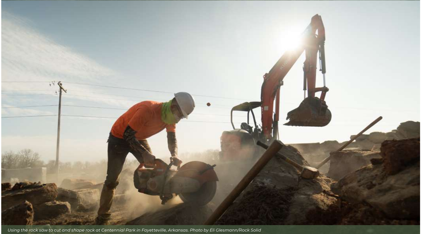
Lots of detailed hand work goes into making rock puzzles secure, stable, and fun. Photos by Chris Guibert/Rock Solid
