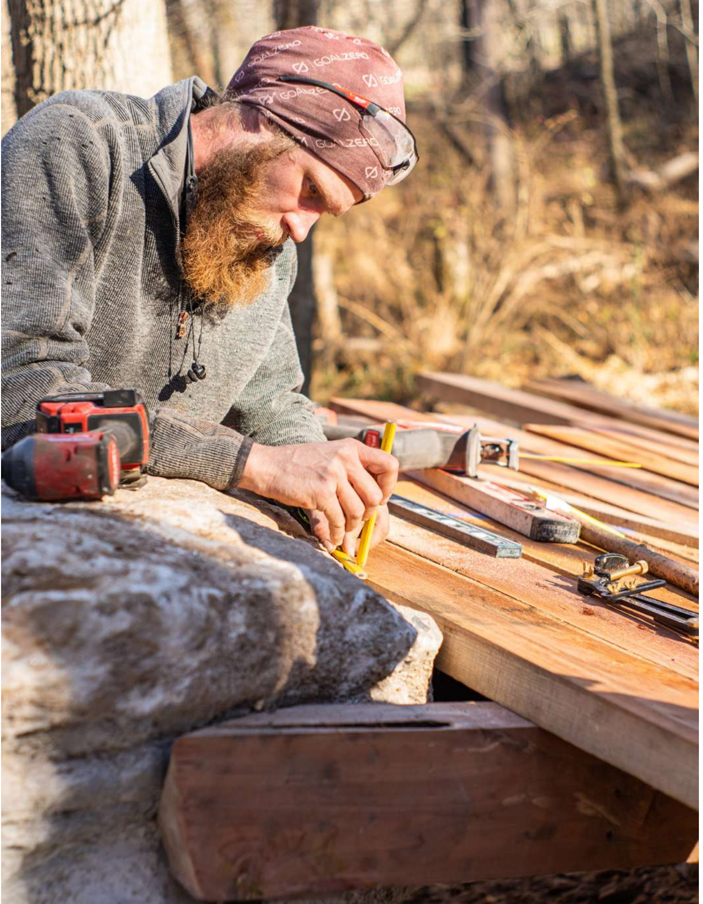
Building a custom wood-stone trail feature at HandCut Hollow in Bentonville, Arkansas. Photo by Eli Clesmann/Rock Solid
