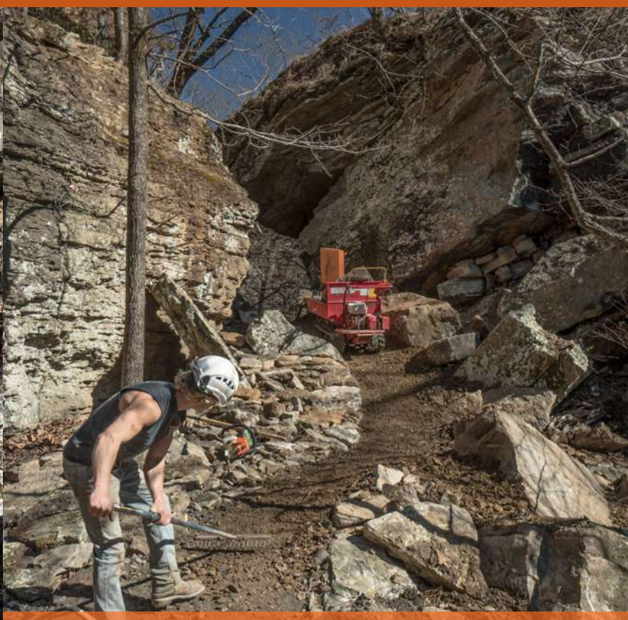
The "after" view of the same rock cliffs and overhang with a new trail routed through the area/point-of-interest. Photo by Eli Glesmann/Rock Solid
