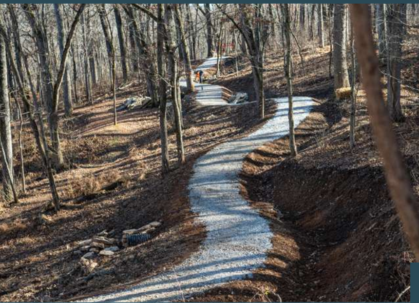
Chip-seal climb trail ready for top coats of liquid asphalt and fine aggregate at Coler Mountain Bike Preserve in Bentonville, Arkansas. Photo by Eli Glesmann/Rock Solid
