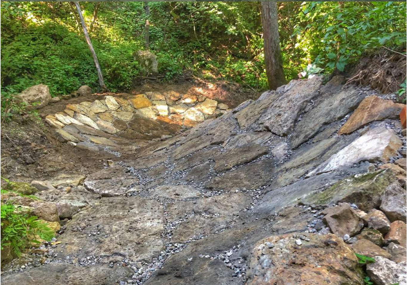
Armored S-berm at Welch Village in Welch, Minnesota. Photo by Adam Buck/Pathfinder Trail Building
