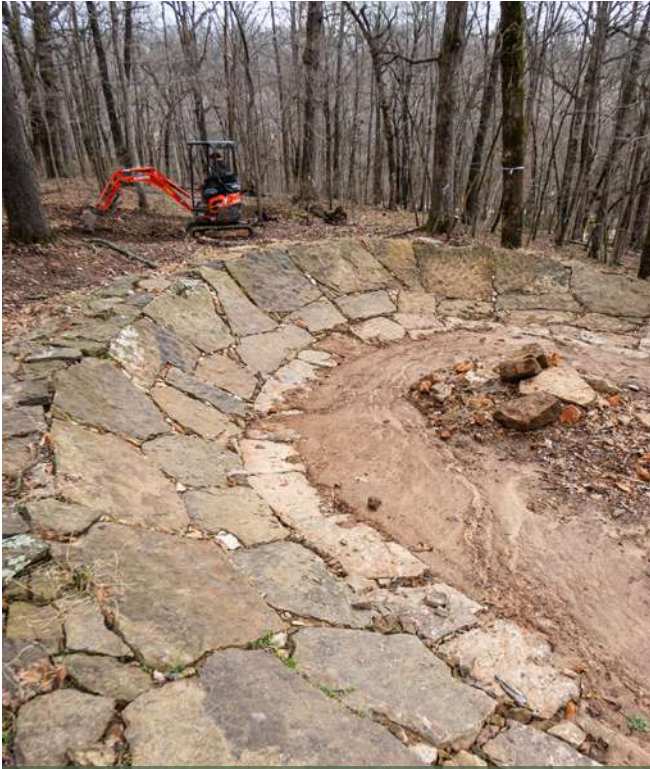
Rock berm under construction on the Boo Boo trail at Slaughter Pen in Bentonville, Arkansas Photo by Kyle Copeland/Rock Solid
