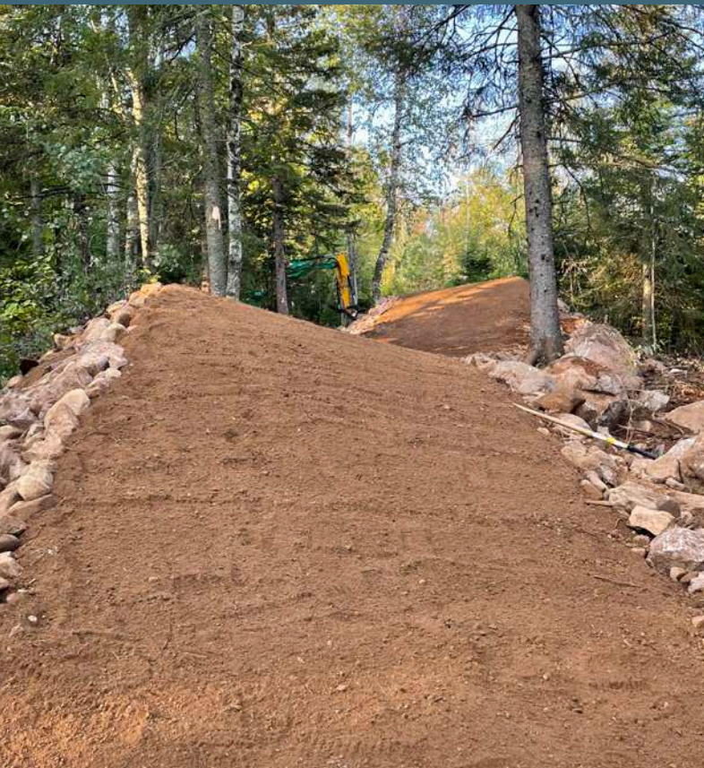
Monster banked berm rollers (brollers!) pre-compaction at Giants Ridge in Biwabik, Minnesota Photo by Adam Buck/Pathfinder Trail Building
