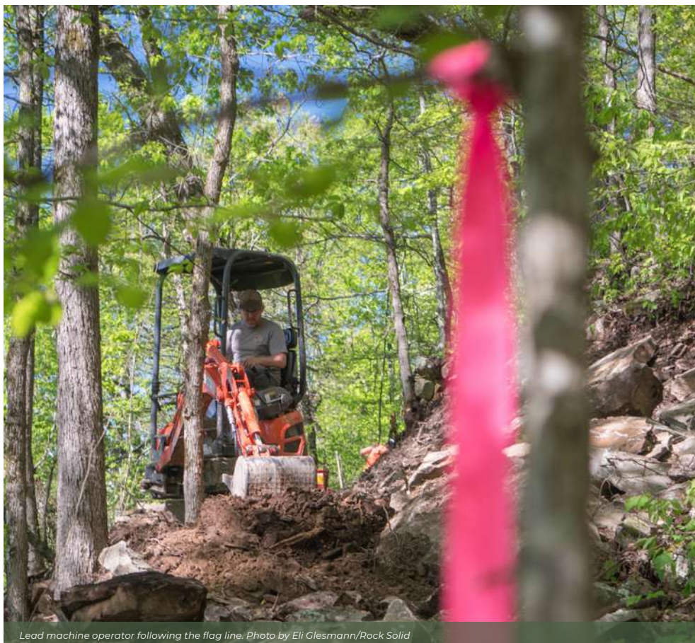
Lead machine operator following the flag line. Photo by Eli Glesmann/Rock Solid
