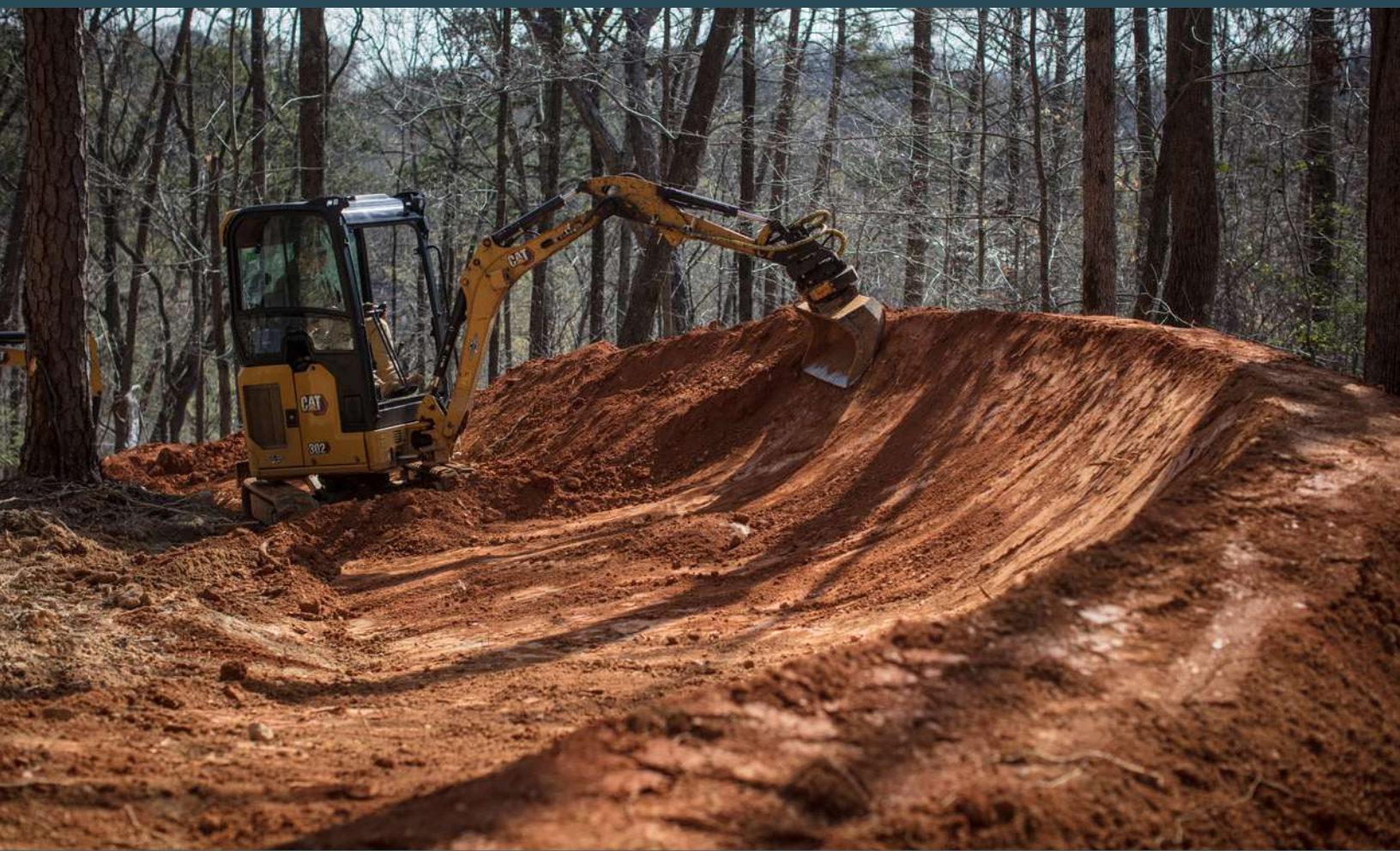
Rebuilding large features with equipment can be beneficial if logistically feasible. Photo by Chrisman/IMBA
