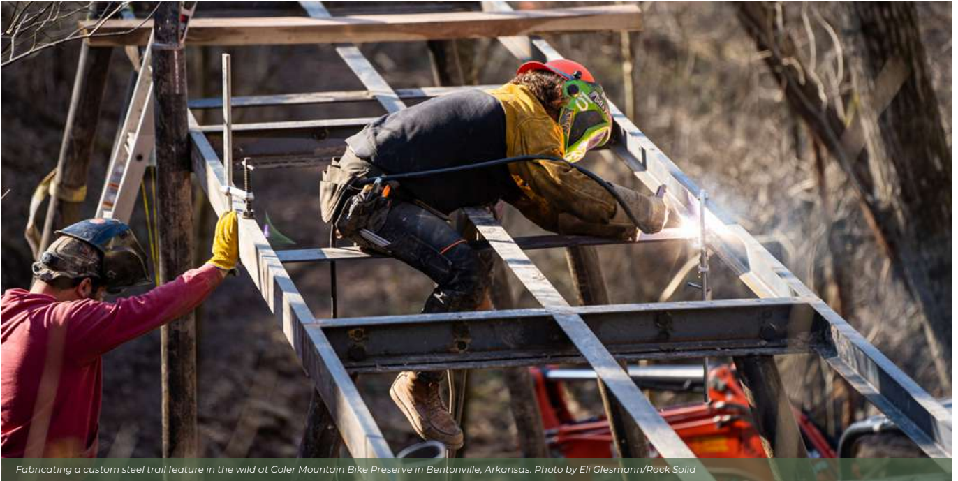
Fabricating a custom steel trail feature in the wild at Coler Mountain Bike Preserve in Bentonville, Arkansas. Photo by Eli Glesmann/Rock Solid
