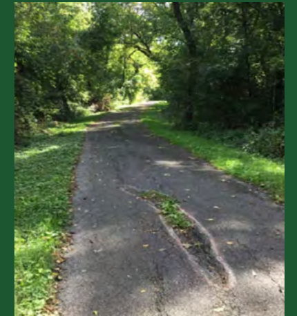
Example of poor condition trail on the Erie Canalway Trail/Empire State Trail in Utica, NY. Source: Hudson River Valley Greenway Empire State Trail Inventory of Existing Trail Sections Report (2020).
