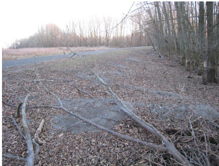
Figure D.19. Displacement of surface aggregate due to water.
