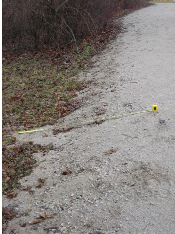
Figure D.8. Water displacement of the surface aggregate.
