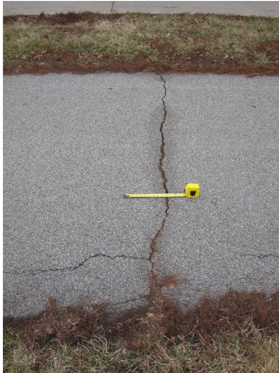
Figure D.13. Typical thermal crack.
