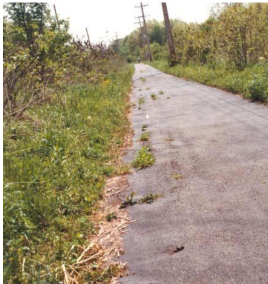
Figure 7. Pop-ups through the HMA layer (ODOT).
