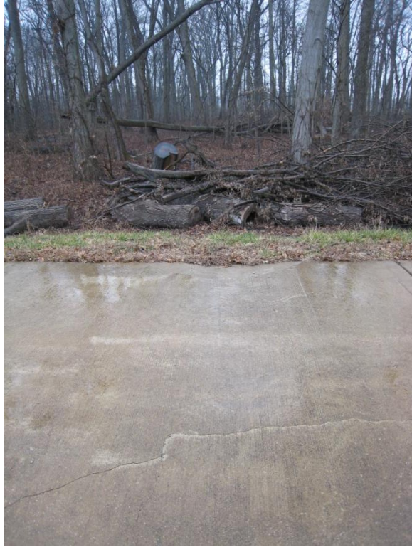
Figure D.25. Slab shattered by tree removal equipment.
