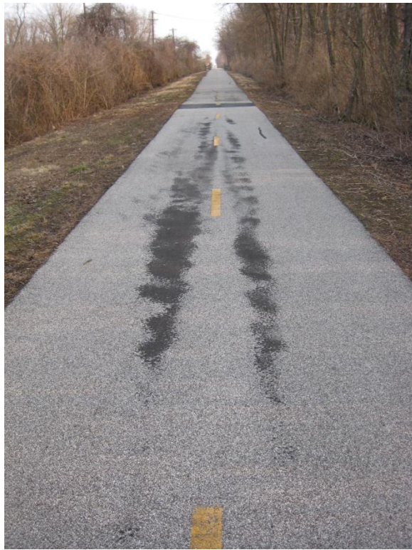
Figure D.40. Localized binder bleeding.
