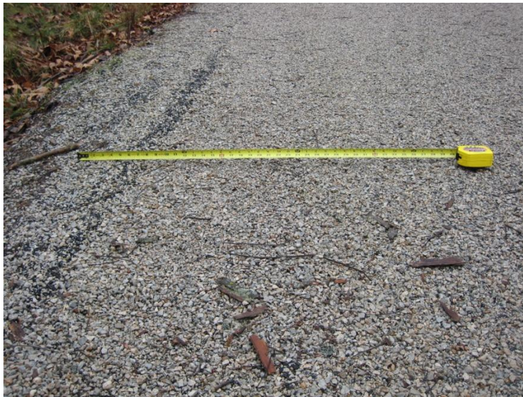
Figure D.11. Grade variation in the bituminous surface treatment.
