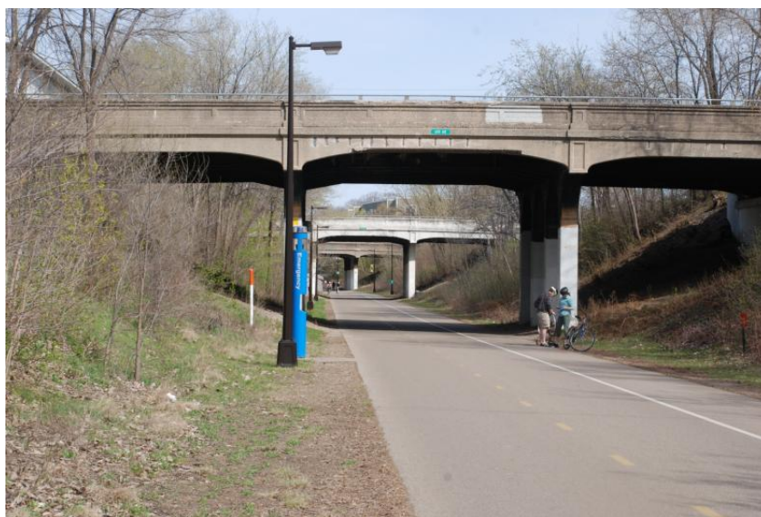
Photo 1 - The Trench of the Midtown Greenway stretches from Hennepin Avenue to 28 th Avenue, with many ramps and staircases to the street network above but only one at-grade crossing (photo by the author, 2010)
