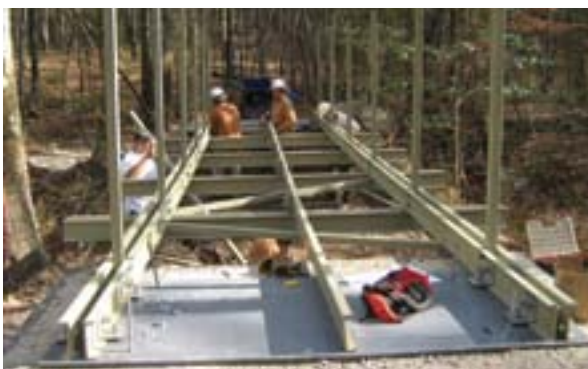
Any delay in material delivery, project sequencing, or weather could impede the completion of this major structure and perhaps other trail or project work.
