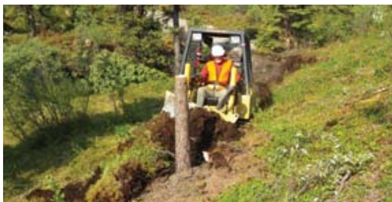
The dozer is removing the organic layer of vegetation and grubbing stumps. Note the high-cut stump for increased visibility and leverage.
