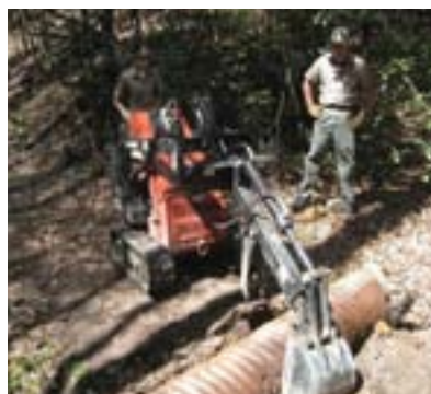
Removing culverts reduces maintenance, restores natural hydrology, provides a dip for trail drainage, and improves aesthetics.
