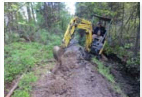
A ditch is being cut along this trail to drain the trail tread and intercept water seeping out of the inside bank. Note that the excavated material is being used to raise the elevation of the trail tread.
