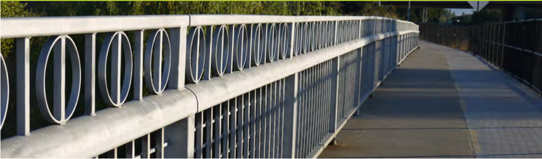
TUBULAR STEEL FENCING
