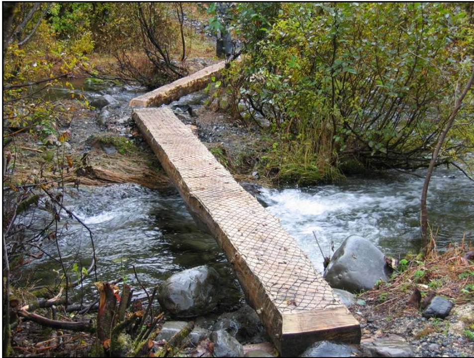
Single span trail bridge. Actively flowing water during heavy rains poses potential safety risk.
