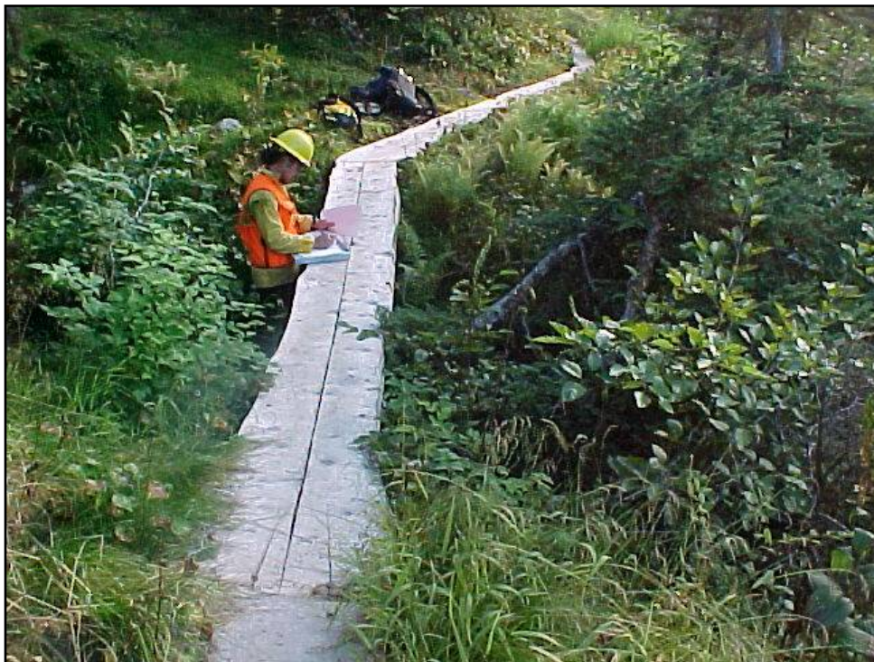
Structure has all the basic structural elements. It is 3½ feet above an active channel.
