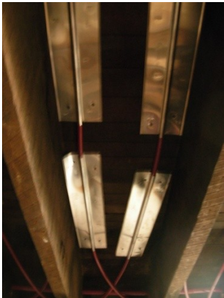
Floor Tubing And Panels
