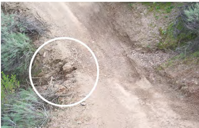
Figure 3–16. Headcut starting from water leaving the trail at too high of a velocity and creating a waterfall effect. Los Padres National Forest, California. USDA photo by Scott Johnson.
