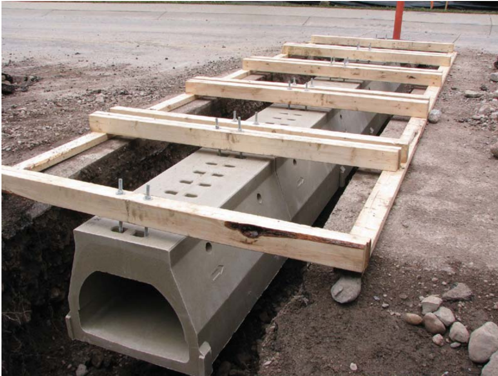
Figure 55. Photo. Construction and placement of amphibian tunnel in Waterton National Park, Alberta (Credit: Parks Canada).
