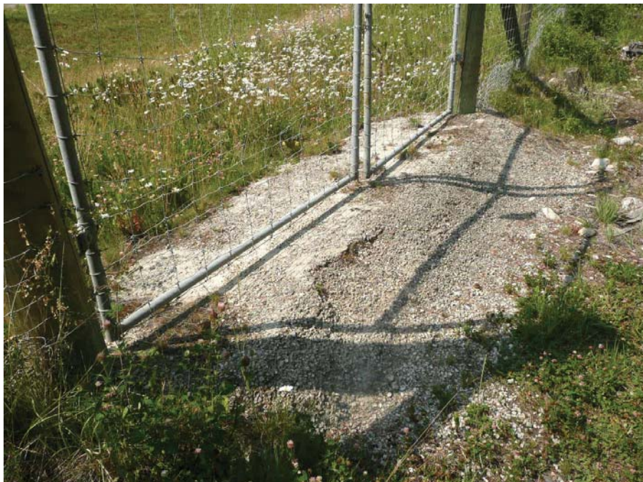
Figure 66. Photo. Concrete base of swing gate to prevent animal digging under wildlife fence (Credit: Tony Clevenger).
