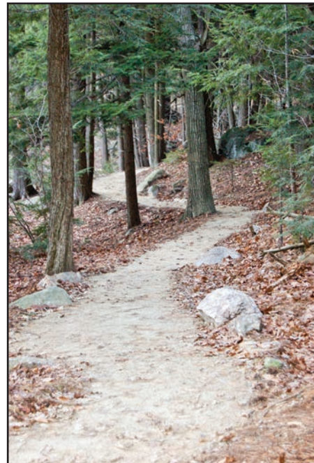
Figure 128—Natural materials were used to build a firm and stable surface for the Crotched Mountain Trail in New Hampshire.
