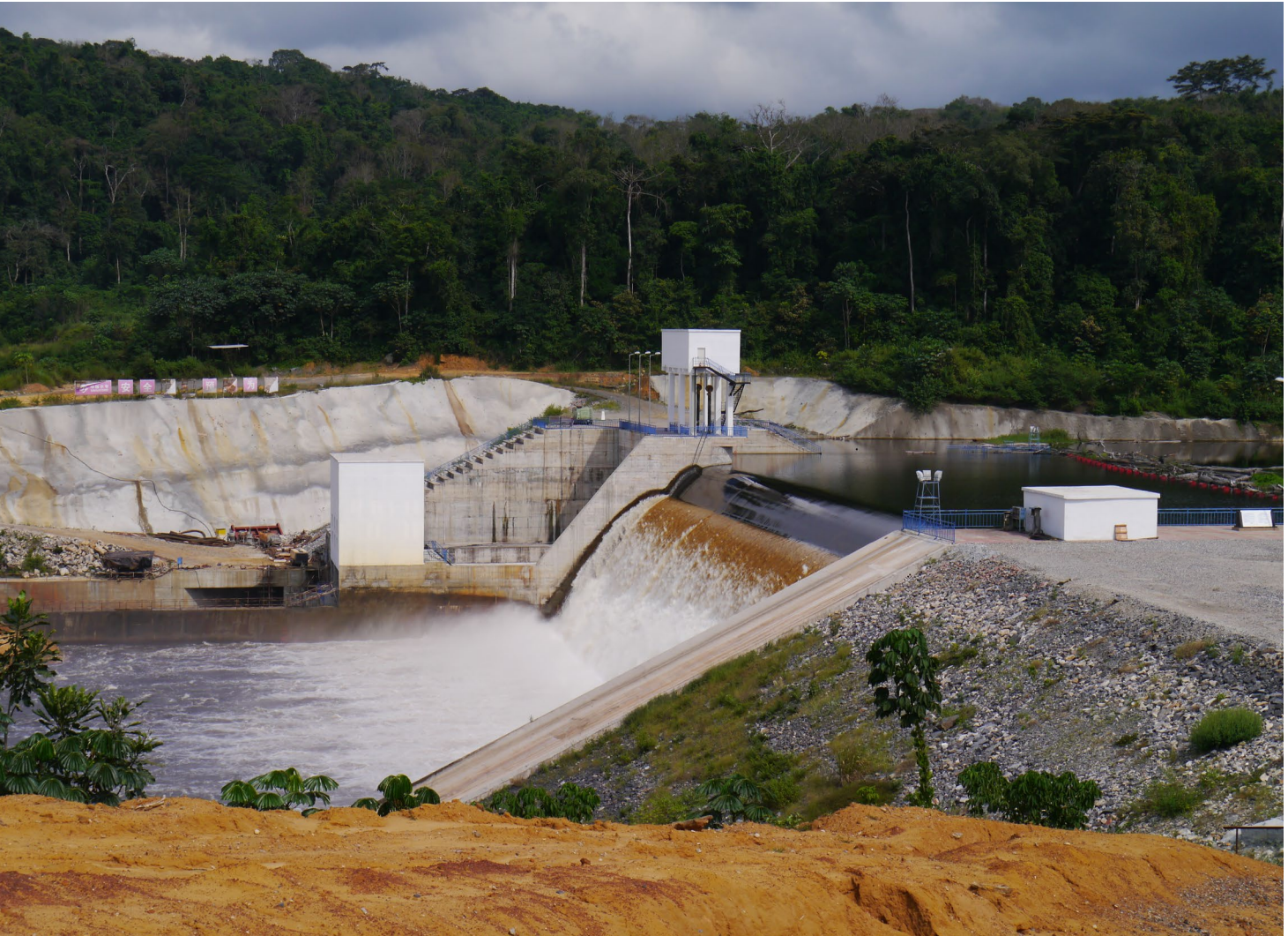
Dam construction tends to have substantial environmental and social ramifications. Grand Poubara dam, Gabon. © Marie-Claire Paiz/TNC
